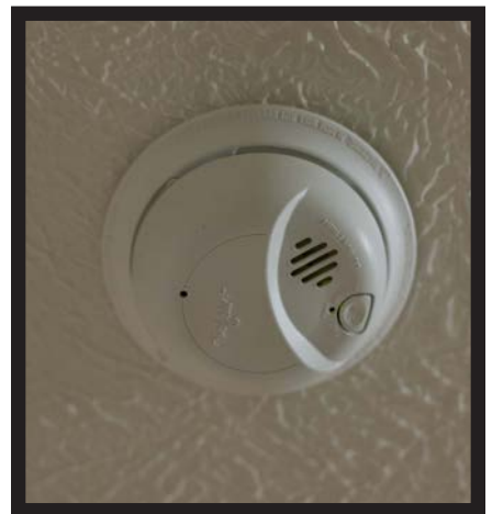
Smoke Detector Carbon Dioxide Detector
