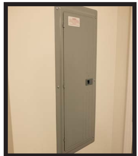
Upgrade Panel Box (20/40 ilo 16/32) - 200 AMP Service (grey cover ilo white)
